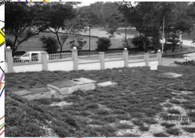
Greywater Reuse System
